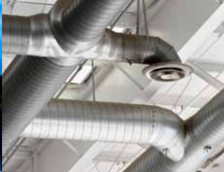
Aquaheat New Zealand Limited: Ventilation and Air-conditioning
